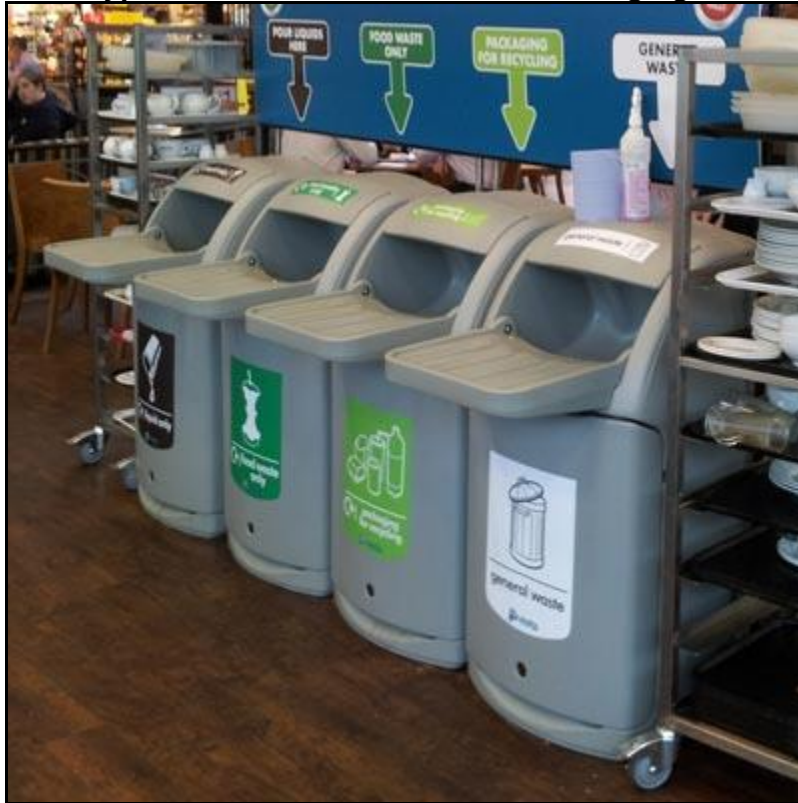
Figure 1 Typical Canteen / Kitchenette waste segregation bin system
